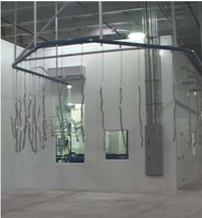
The environmental room controls the heat and humidity for precise application control.
